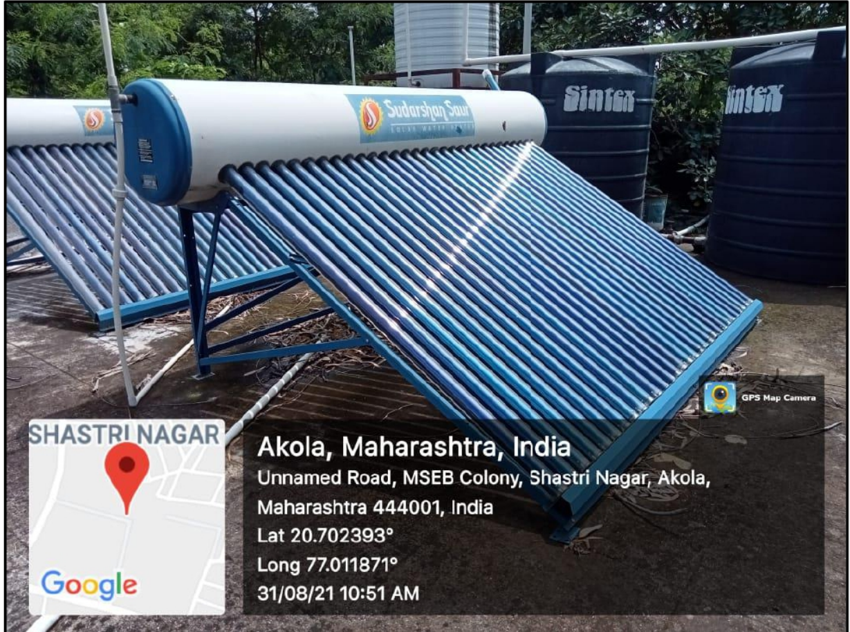
Solar Energy Point 1 & 2
