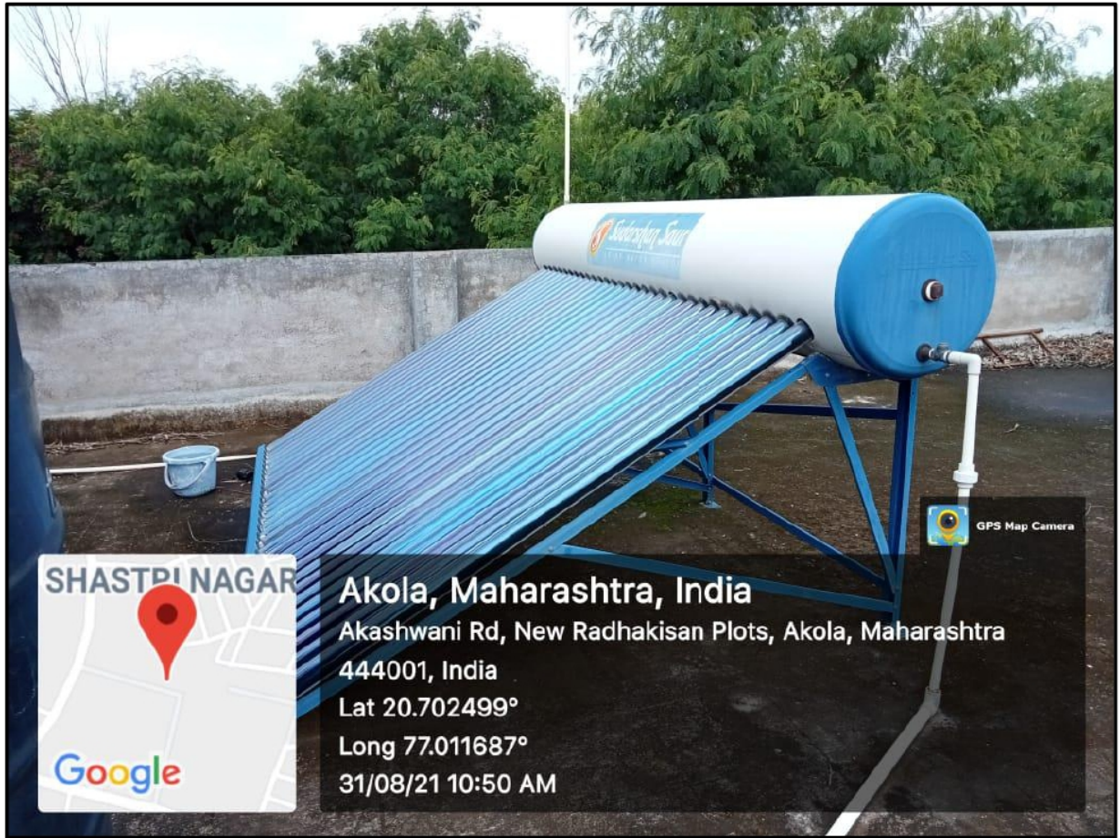
Solar Energy Point 3
